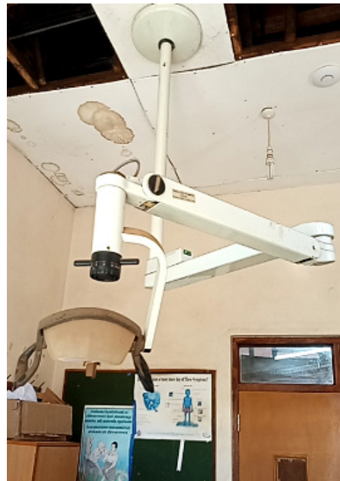
22MW, #083 Ceiling mounted light not used in over 6 months, light does not switch on and safety concerns exist.
