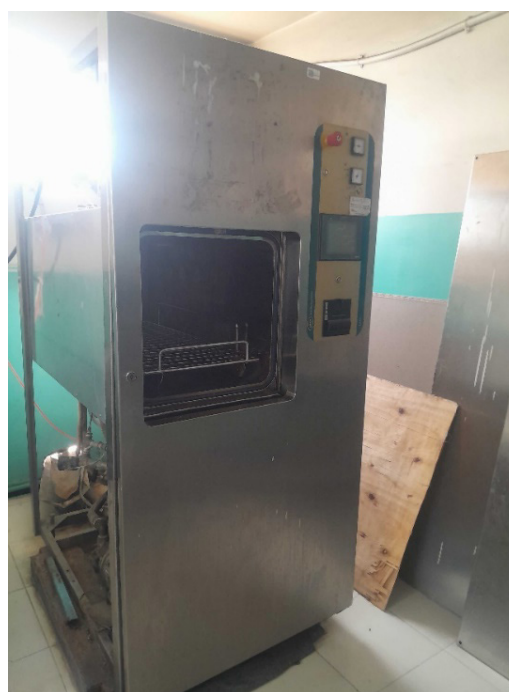
04ET, #123 Although engineers reported this autoclave met all of the benchmark compliant criteria, they noted in the comment section that this machine does not heat. Accordingly, this 4 OR tauma care hospital in the capital is operating without a suitable autoclave.
