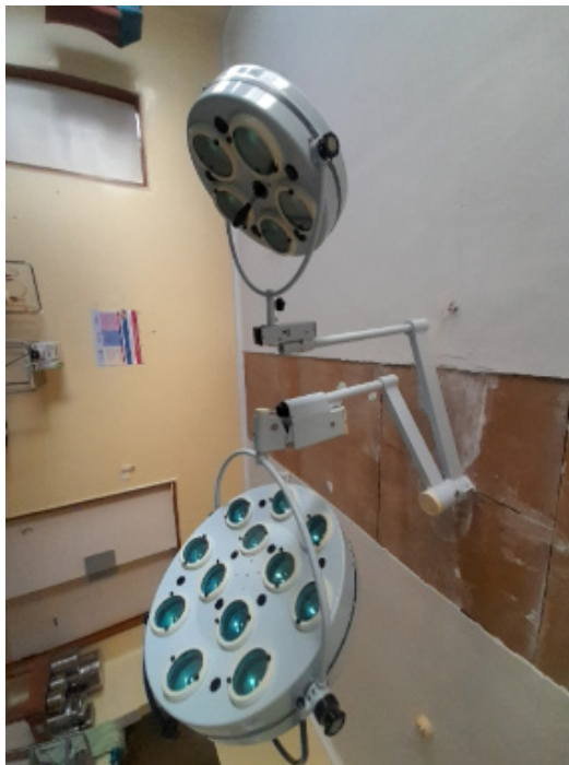
14ZM, #006 Ceiling mounted light used within the past 7 days, with no safety concerns. The equipment is unsatisfactory and all the lights do not work.
